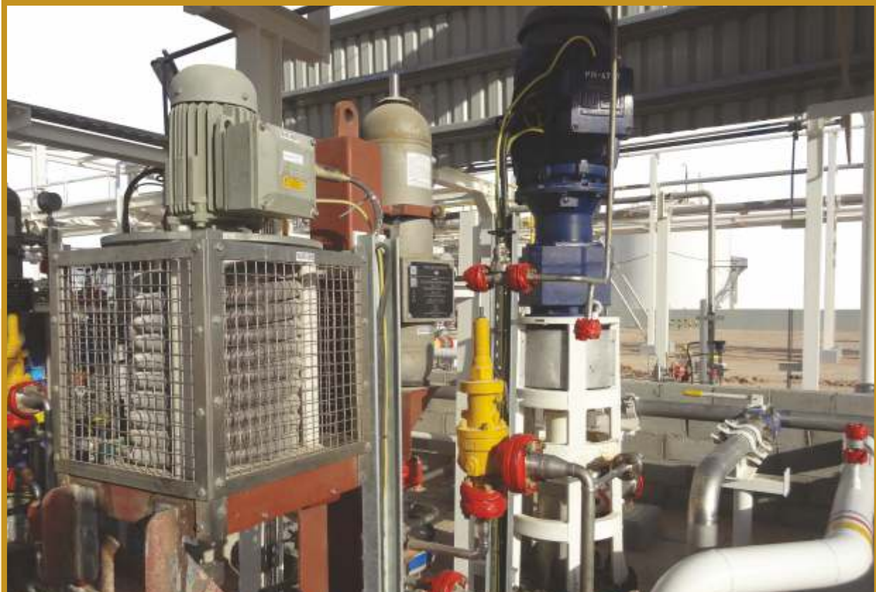
ROTO VMAB 662 PROGRESSIVE CAVITY PUMP TRANSFERRING OIL & WATER MIXTURE AT GROUP GATHERING STATION Duty Point : 42 m 3 /hr @ 4.5 bar
