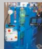
Feeding oily water for separation
